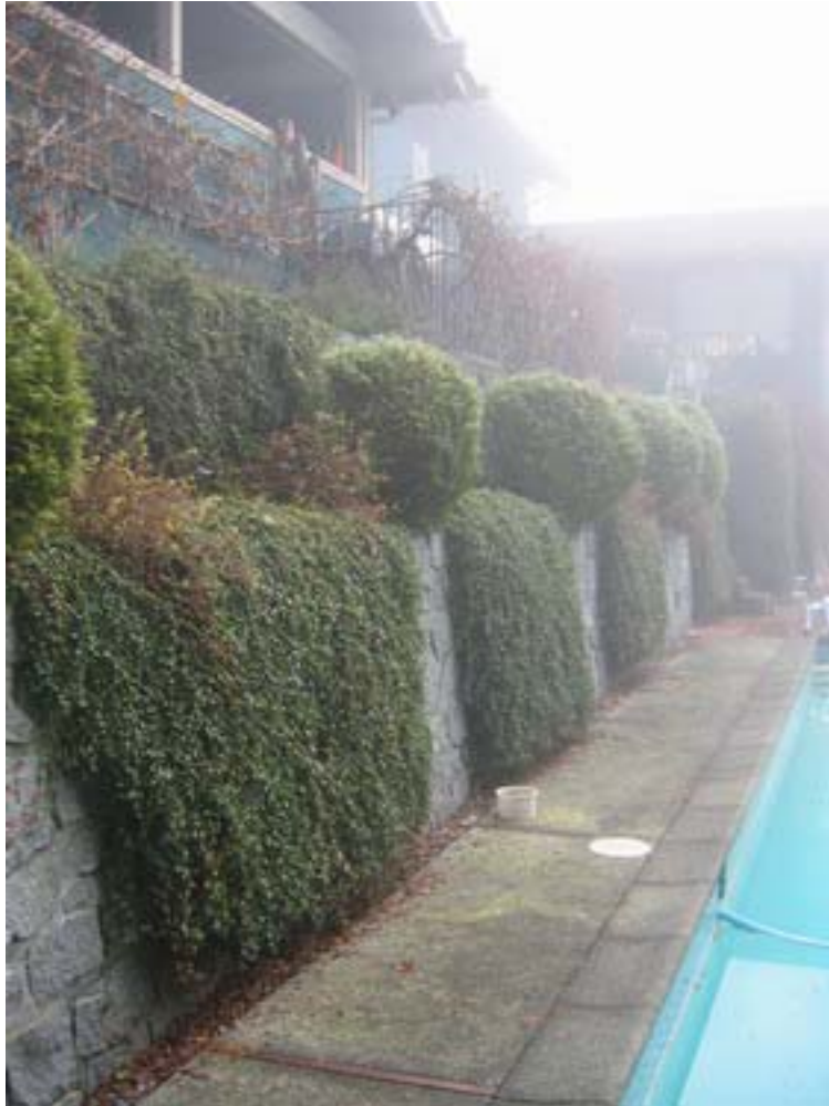
Figure 3. 2379 Carman Place – Concrete and rock retaining wall between the house and pool
