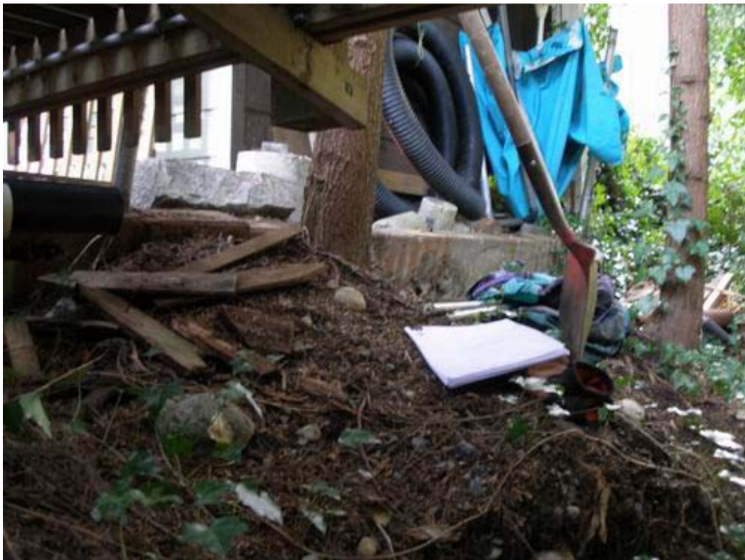
Figure 2. 2474 Hayseed Close – Tilted concrete retaining structure
