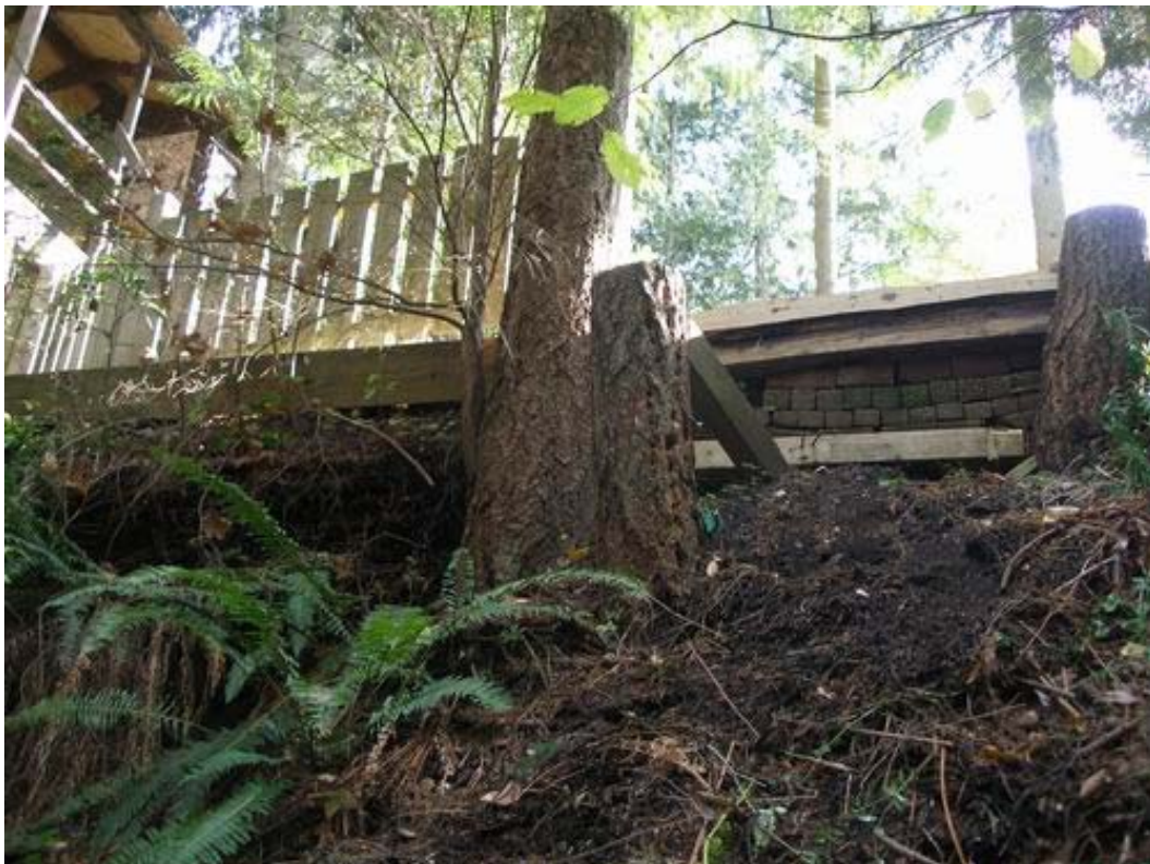
Figure 2. 2486 Hayseed Close – View looking south towards a slumping brick retaining wall
