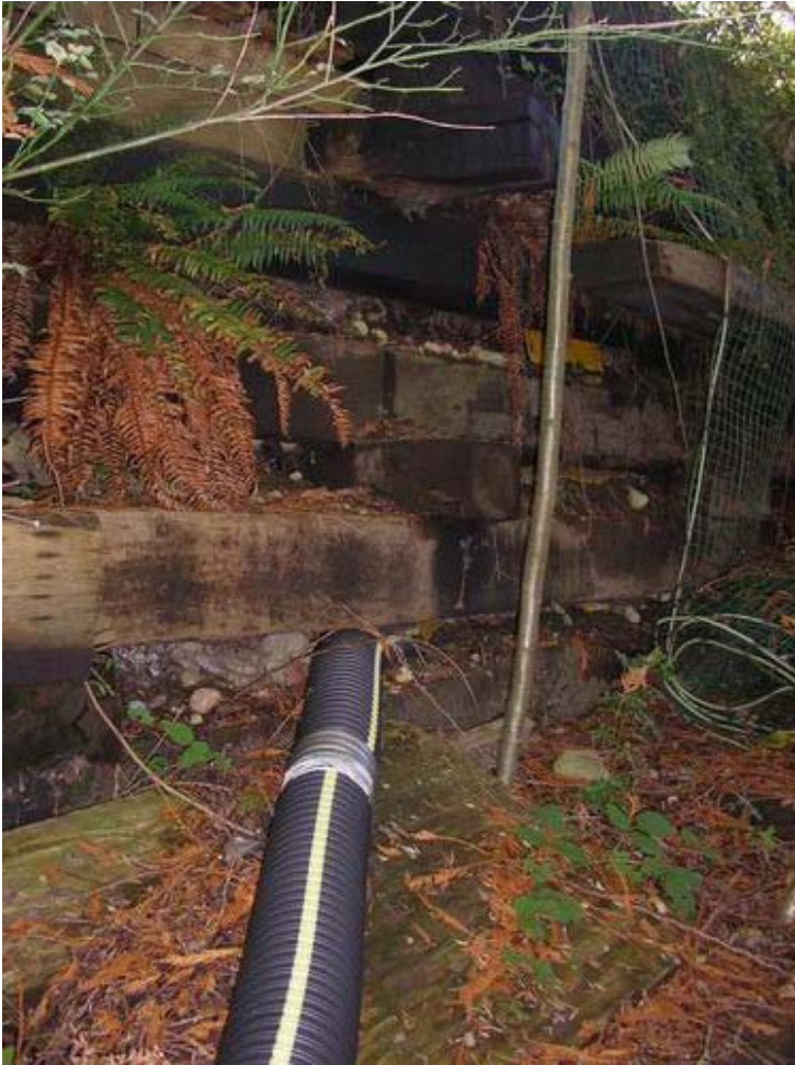
Figure 3. 2480 Hayseed Close – Timber crib retaining wall with protruding drainage pipe
