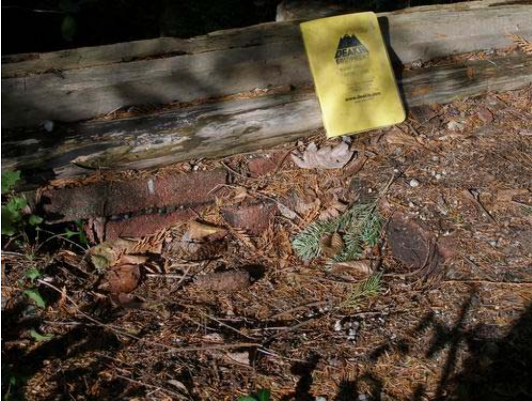
Figure 3. 2486 Hayseed Close – Top view of settling brick retaining wall
