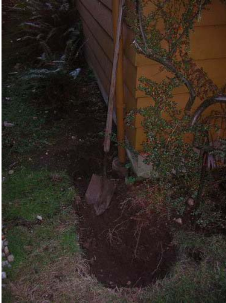
Figure 3. 2125 Berkley Avenue – Pit dug on NW corner of house near roof drain
