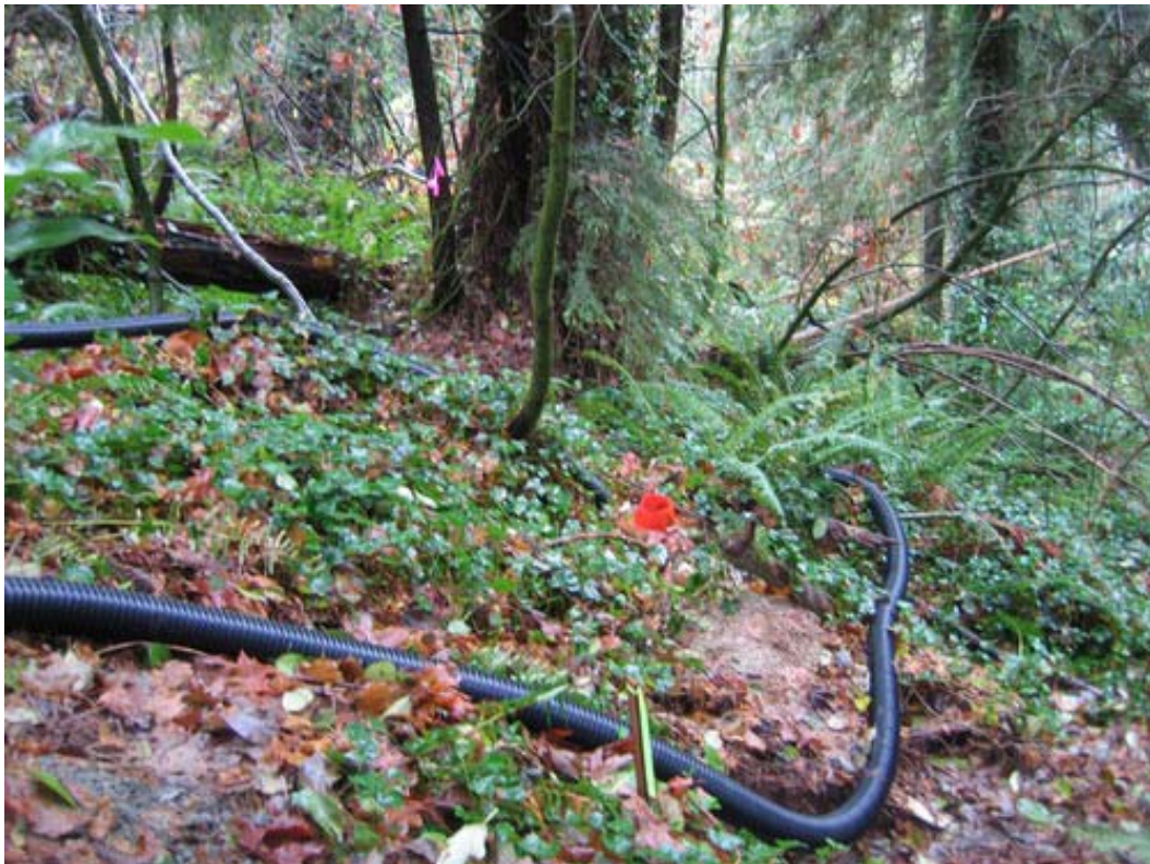
Figure 2. 2223 Berkley Avenue - End of drainage pipes down-slope
