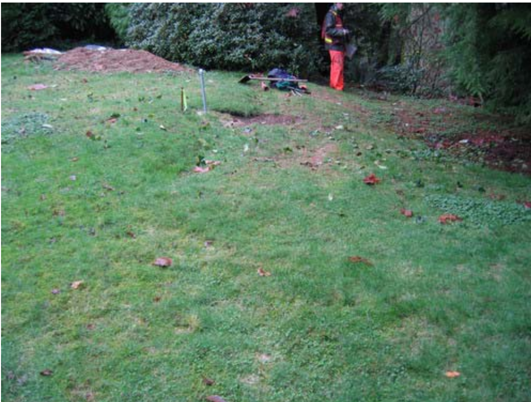
Figure 4. 2223 Berkley Avenue – Slumping in backyard
