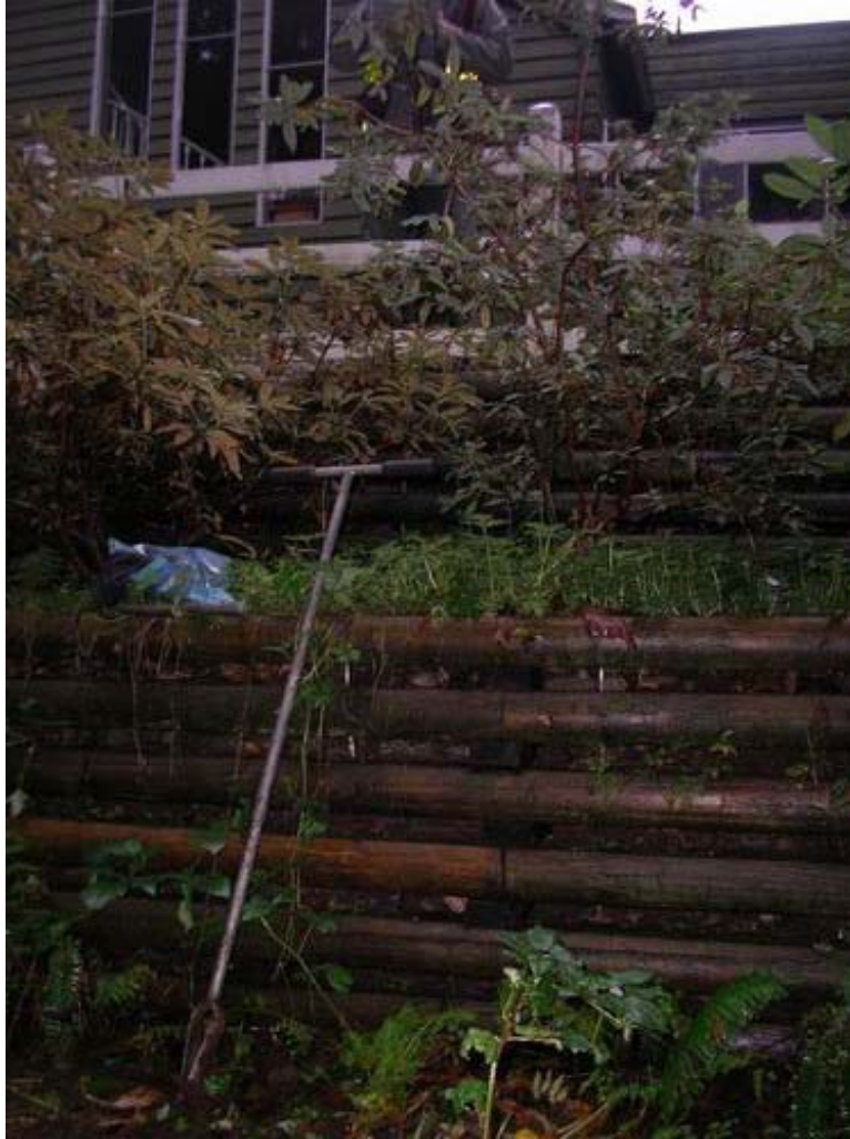
Figure 5. 2265 Berkley Avenue – Two tiers of a four tiered timber crib retaining wall
