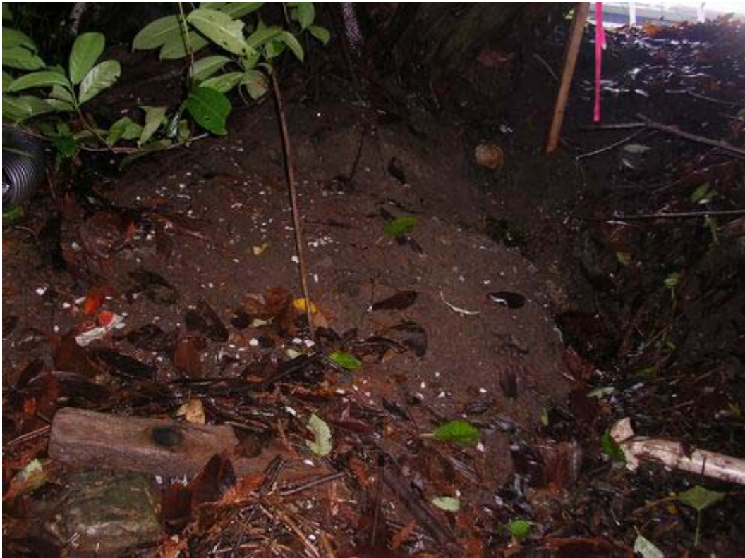
Figure 3. 2265 Berkley Avenue – Significant erosion from pipe draining at crest
