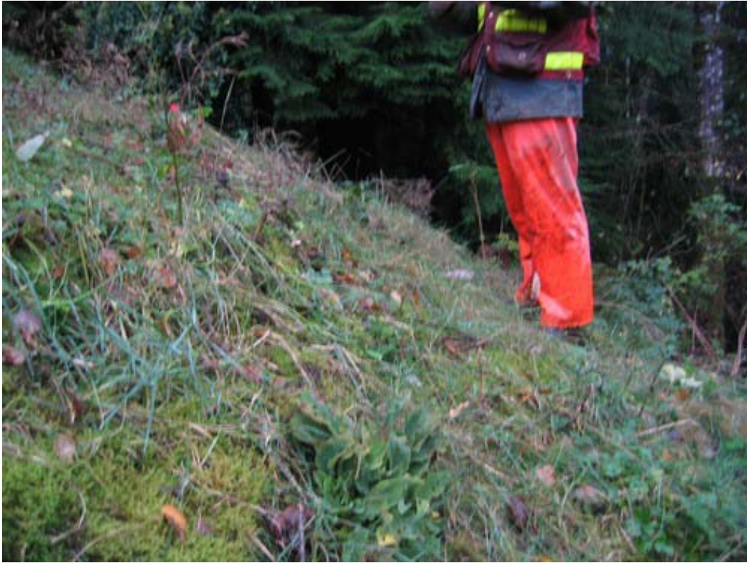
Figure 3. 2293 Berkley Avenue – Slumping near crest of slope
