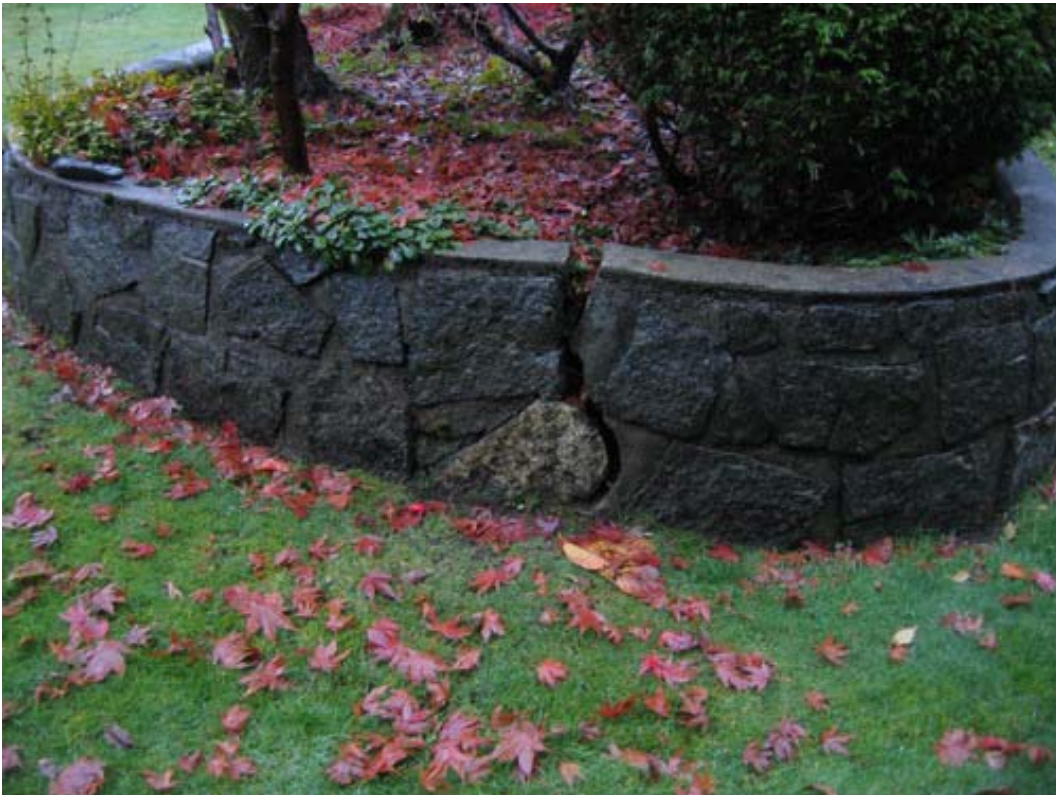
Figure 2. 2293 Berkley Avenue - Cracked planter near slope crest
