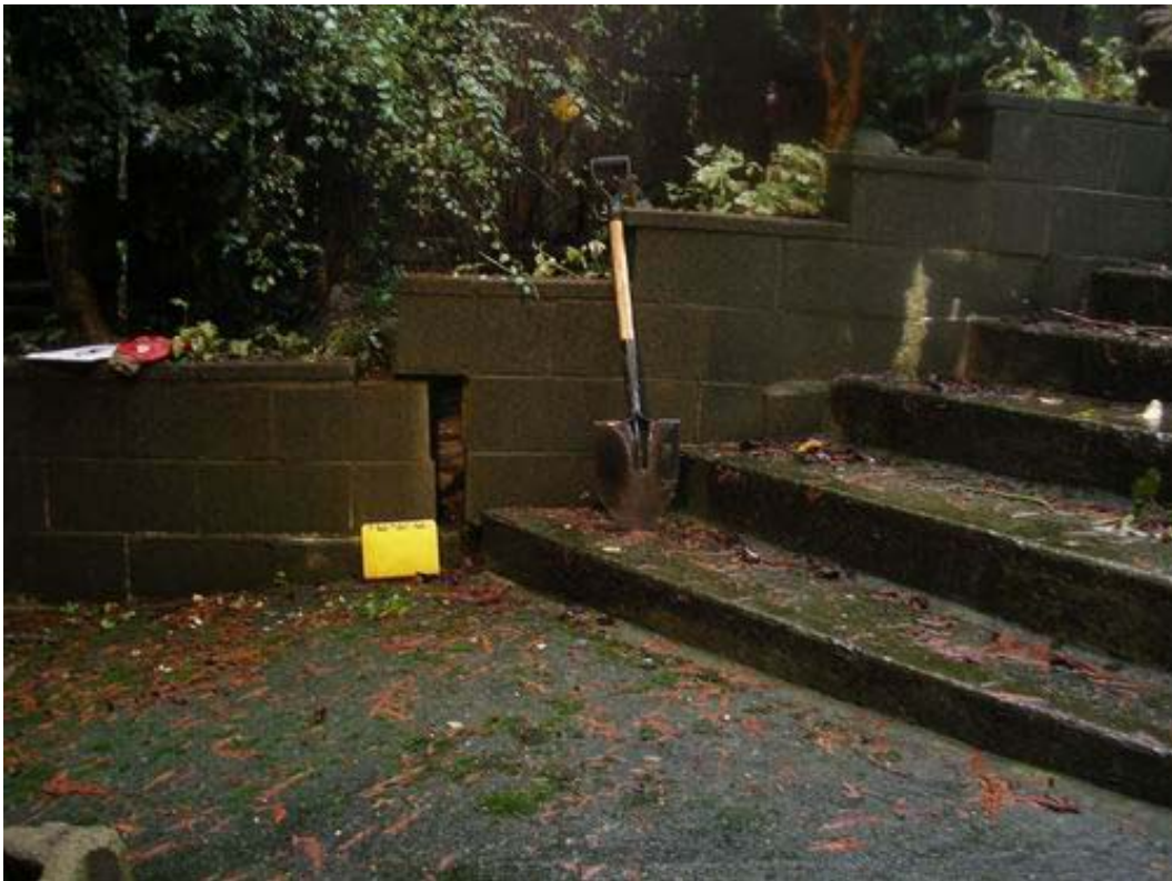
Figure 2. 2265 Berkley Avenue – Large crack in retaining wall
