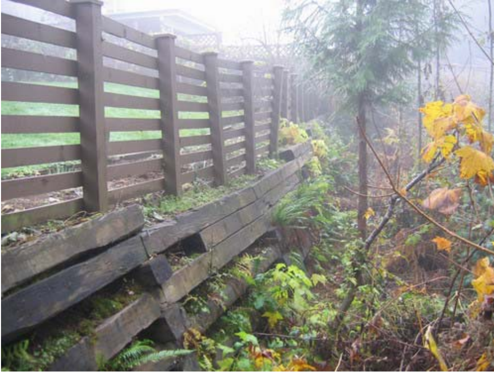
Figure 3. 2321 Berkley Avenue – Settled retaining wall
