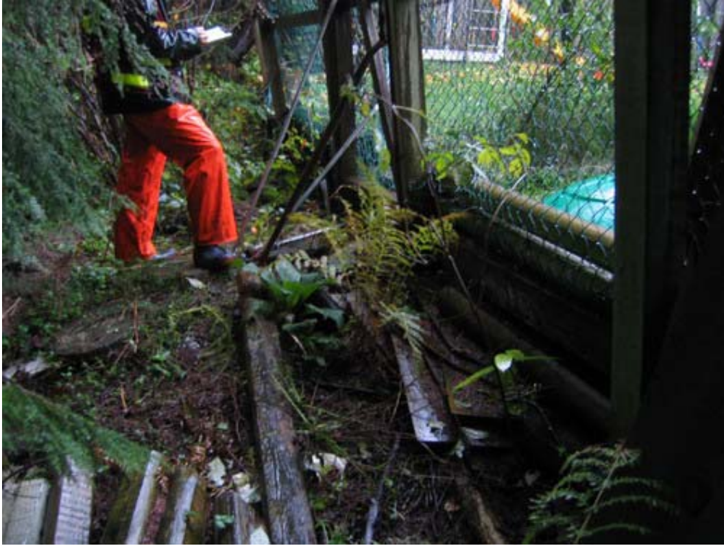
Figure 3. 2349 Berkley Avenue – Retaining wall/fence near crest
