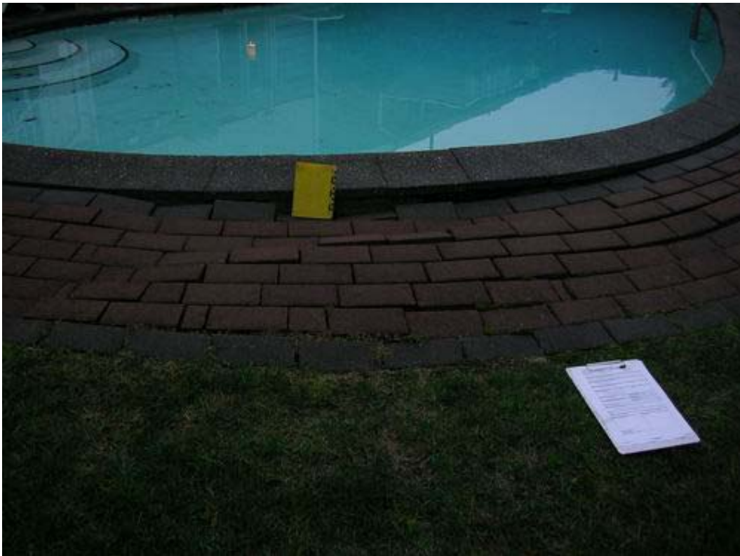
Figure 2. 2307 Berkley Avenue – Settling around pool deck
