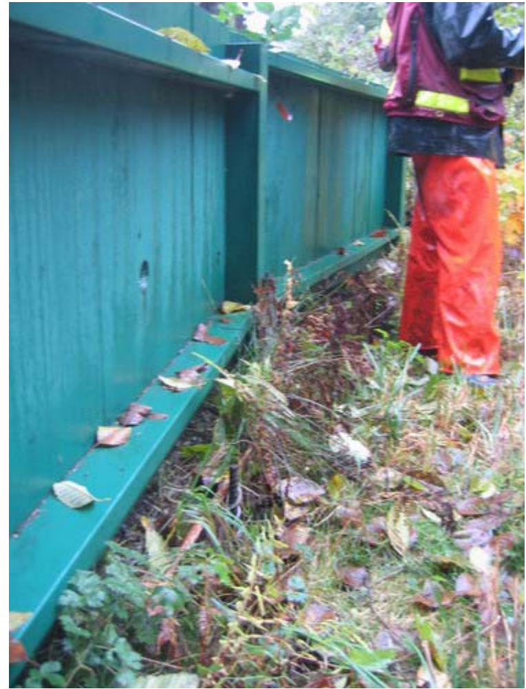
Figure 4. 2391 Berkley Avenue – Retaining wall/fence line and small retaining structures made of rebar and small sticks
