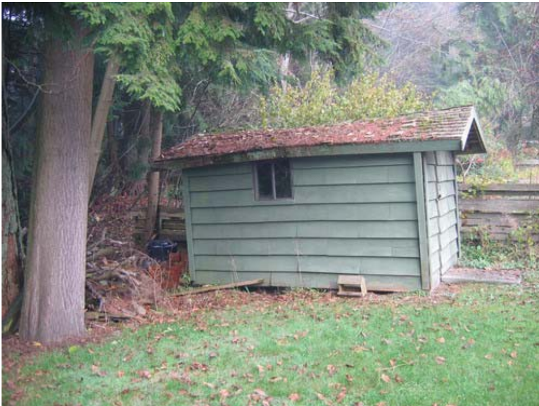
Figure 4. 2425 Berkley Avenue – Shed settling on west side
