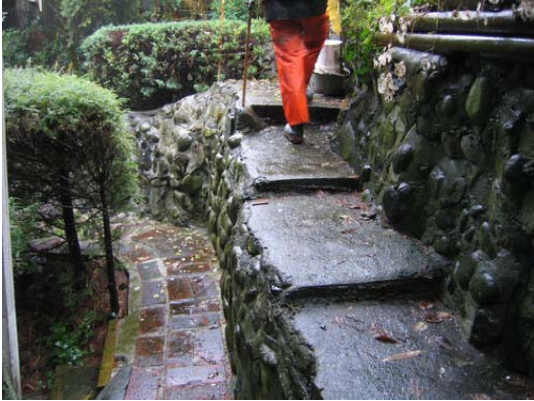
Figure 5. 1305 Lennox Street – Concrete retaining wall above the shed with built in steps
