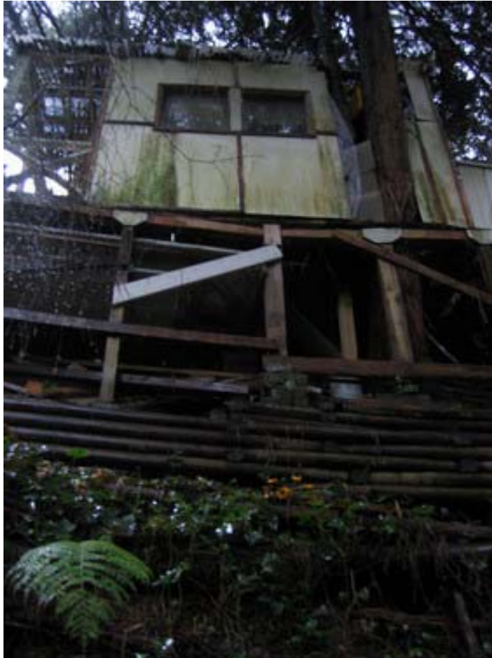
Figure 3. 1305 Lennox Street – Wooden crib wall and shed perched on slope
