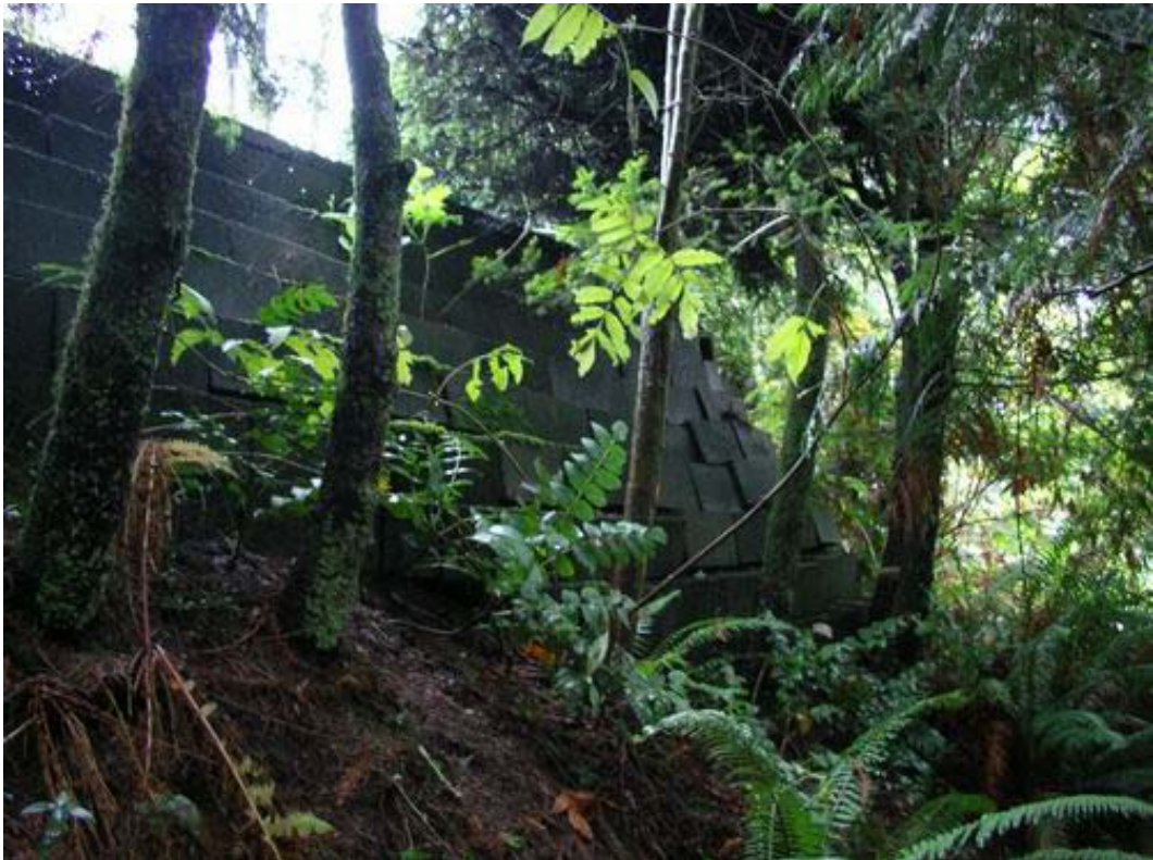
Figure 4. 1231 Lennox Street – Failing concrete retaining wall
