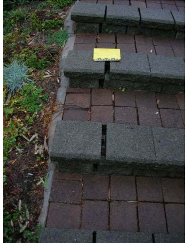
Figure 2. 1383 Lennox Street – Slight deformation in steps
