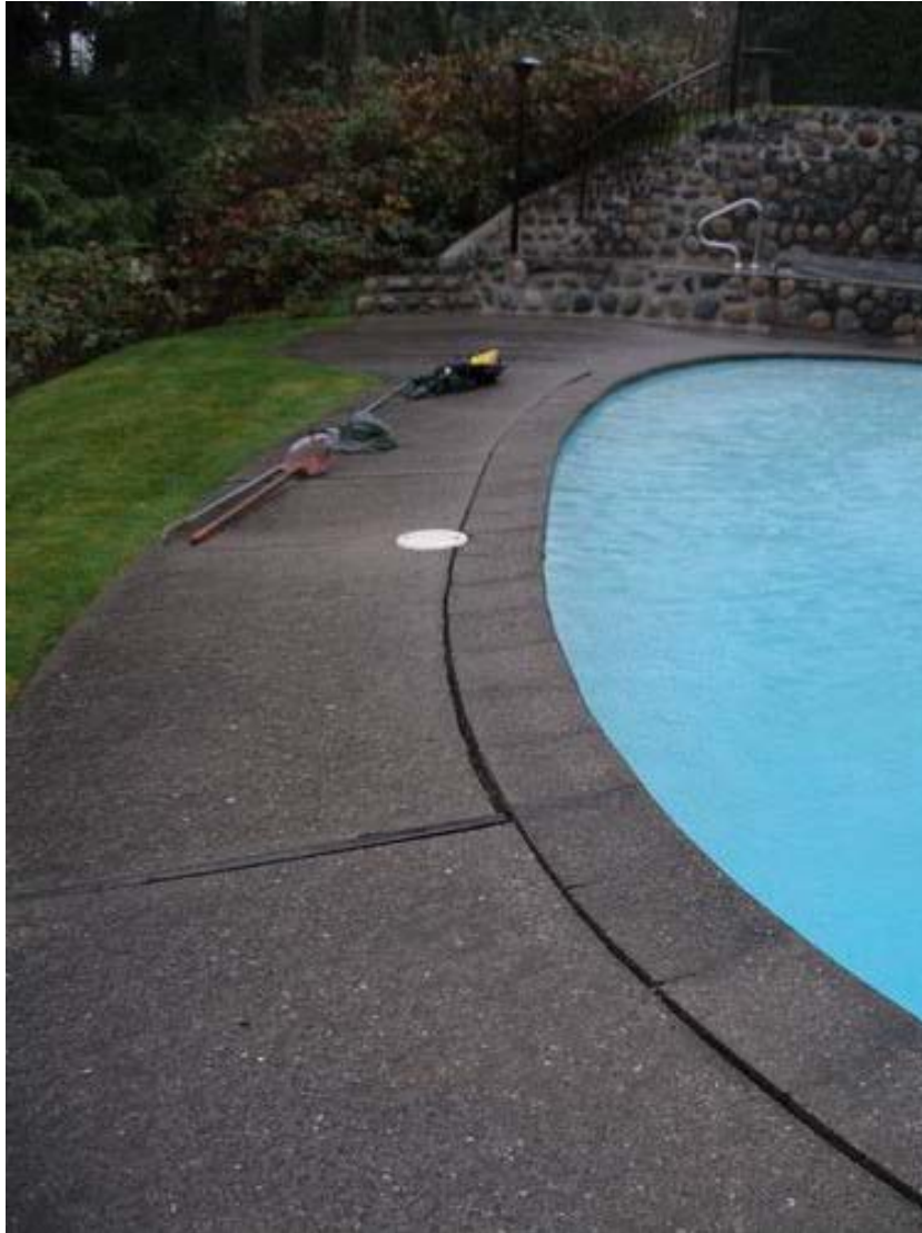
Figure 3. 1425 Lennox Street – Settlement of concrete panels around swimming pool
