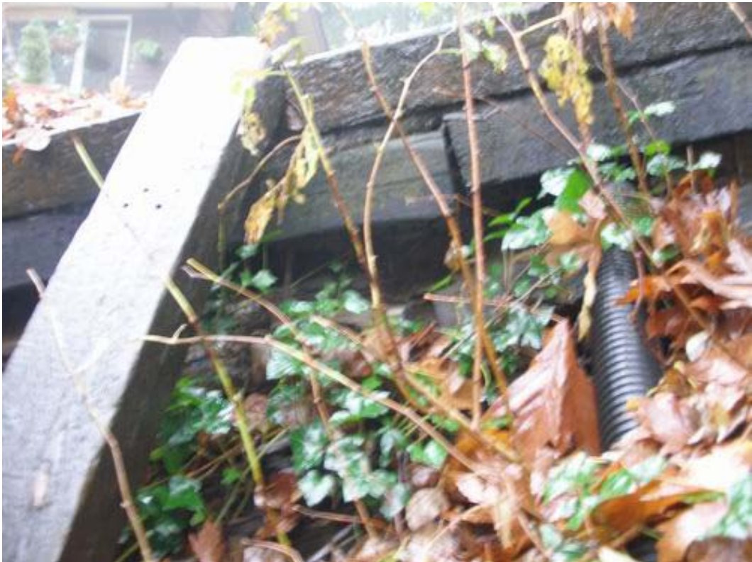
Figure 2. 1535 Lennox Street – Bulging timber crib retaining wall
