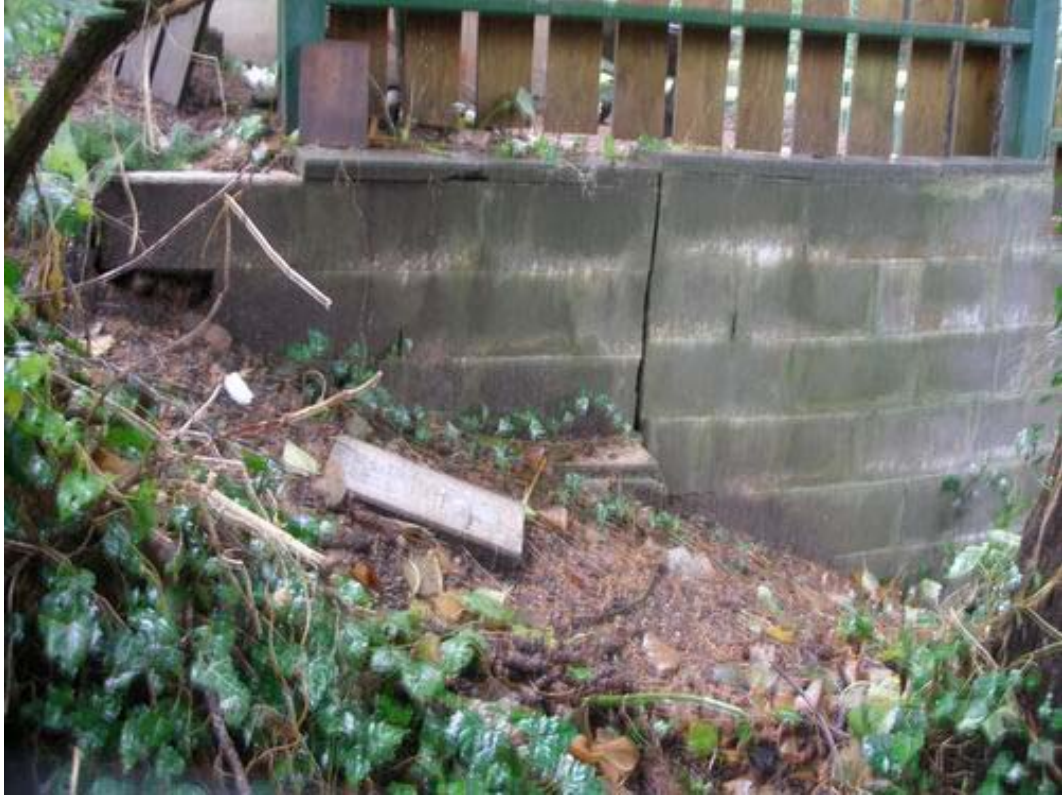
Figure 5. 1593 Lennox Street – Crack on the north side of the concrete retaining wall
