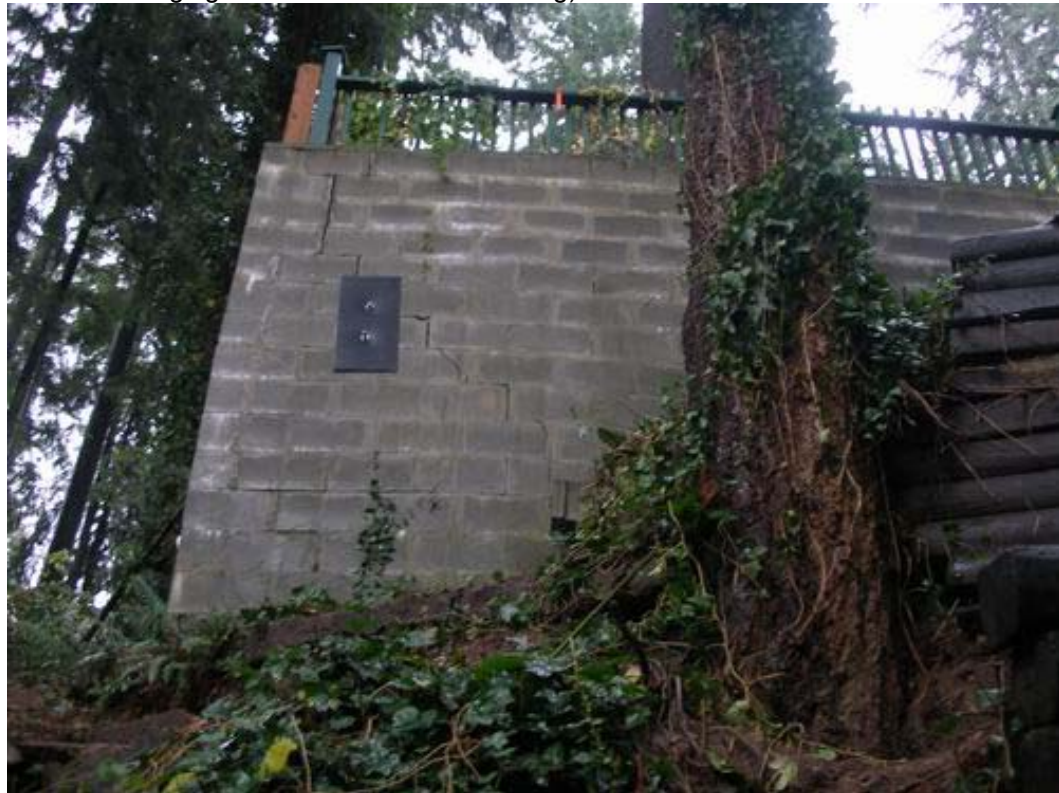
Figure 4. 1593 Lennox Street – Cracking on the west side of the concrete retaining wall
