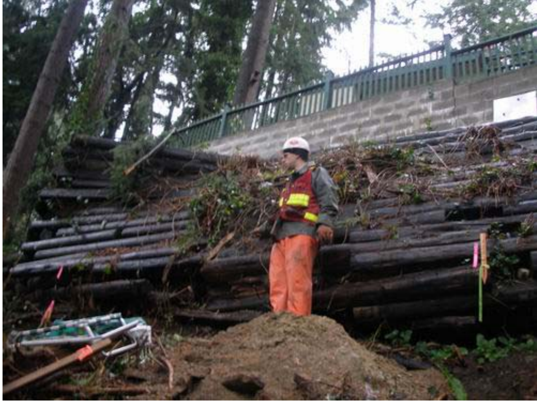
Figure 3. 1593 Lennox Street – Concrete retaining wall built on top of old timber crib wall (timber crib wall is bulging and concrete wall is cracking)
