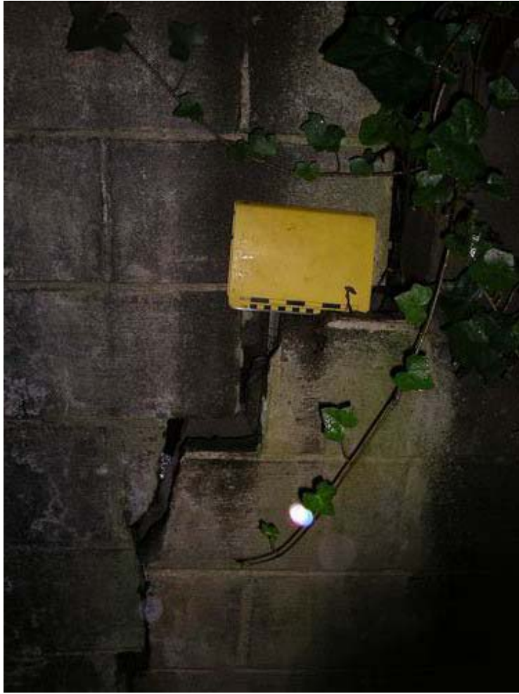
Figure 3. 1557 Lennox Street – Crack in concrete retaining wall
