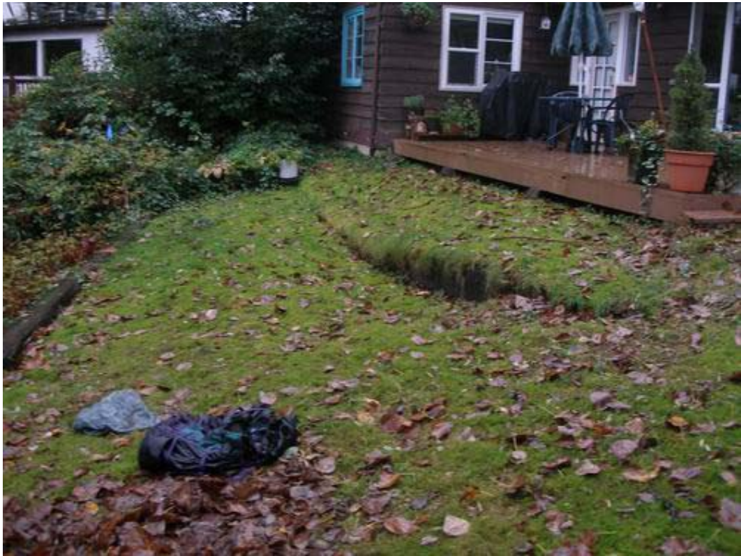
Figure 3. 1535 Lennox Street – View looking north of settling/slumping backyard
