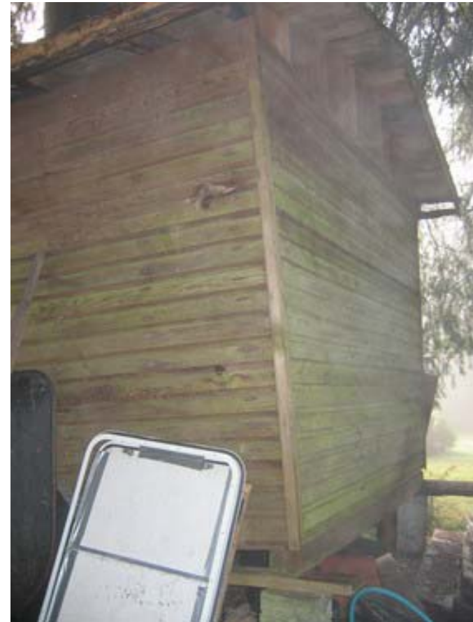
Figure 4. 2414 Swinburne Avenue - View looking south at tilted shed
