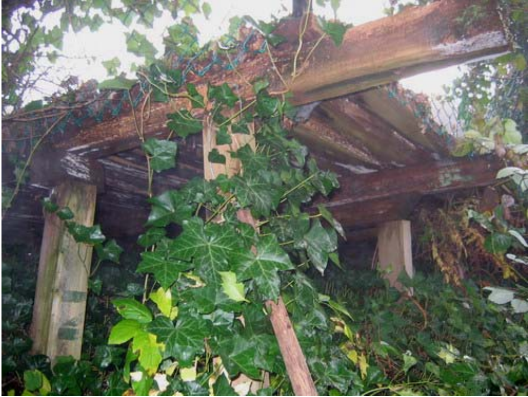
Figure 3. 1731 Layton Drive – View upslope looking at bottom of rotting deck
