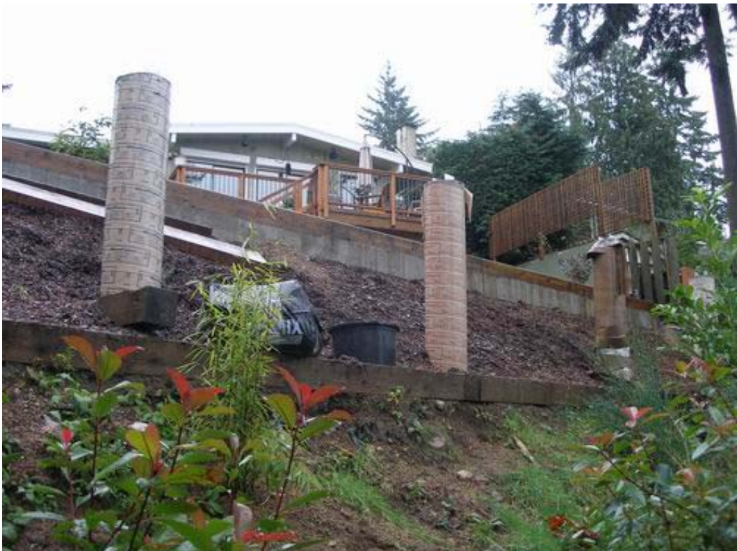
Figure 4. 1815 Layton Drive – View of retaining wall and in-progress construction from west side of property
