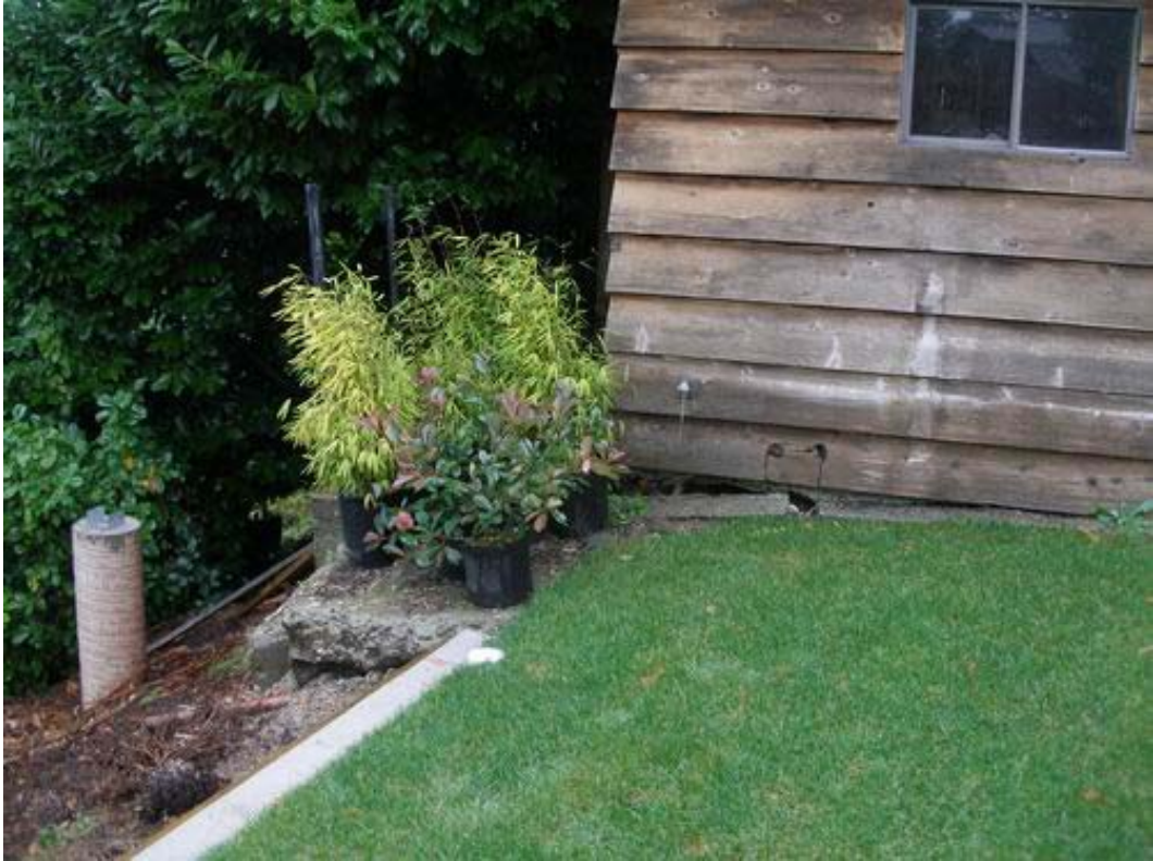
Figure 3. 1815 Layton Drive – Slumping underneath a shed on the NW side of the backyard
